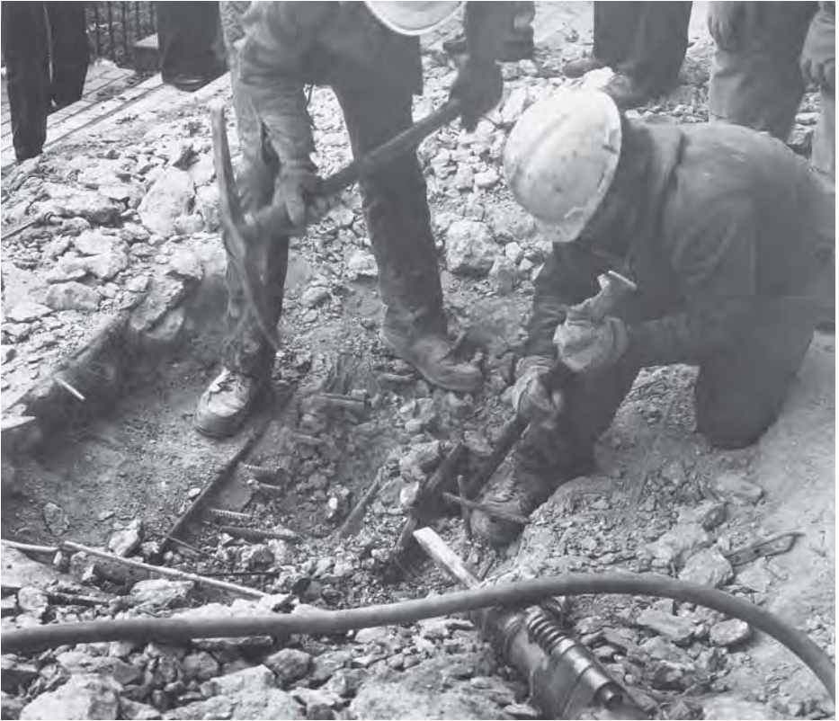
ABOVE: Demolition workers, in December 1987, tear apart the foundation of ALPA's former headquarters building at Midway Airport to uncover a time capsule buried in the front steps.
